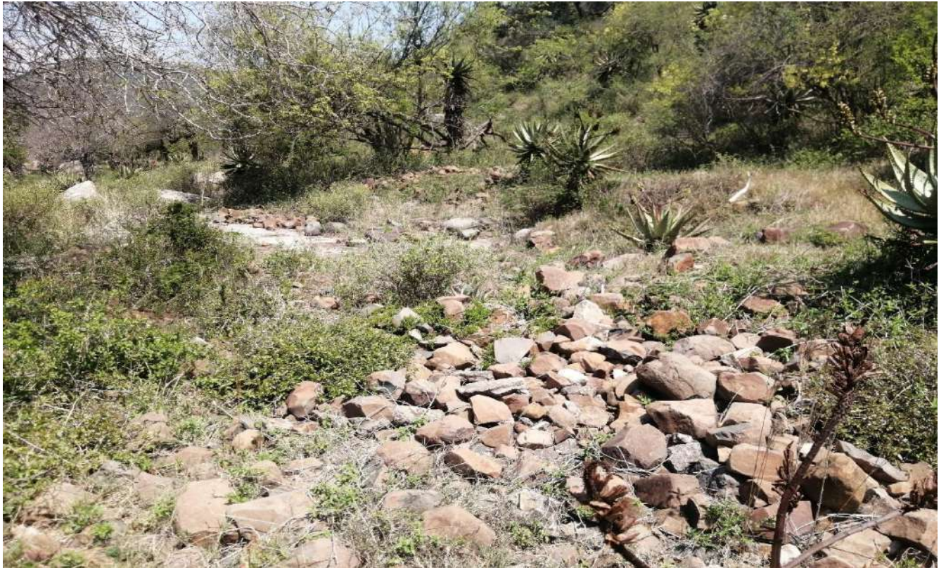
Figure 31: Showing collapsed stone walling near derelict dip tank identified on site MHB01.
